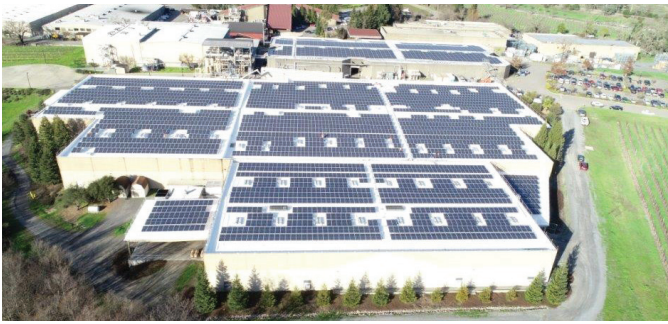
SPF roof with photovoltaic panels at the Rodney Strong Vineyards in Healdsburg, CA.
