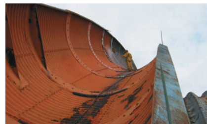
Previous repairs to the roof were not successful in keeping the leaks away.
