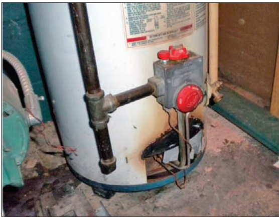
Evidence of flame roll-out.
